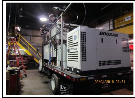
Photo # 2 View of DCI Dry Fog Truck during assembly with fog nozzles on top
