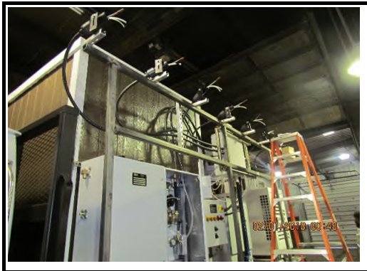
Photo # 5 DCI Dry Fog control panel with fog nozzles on top
