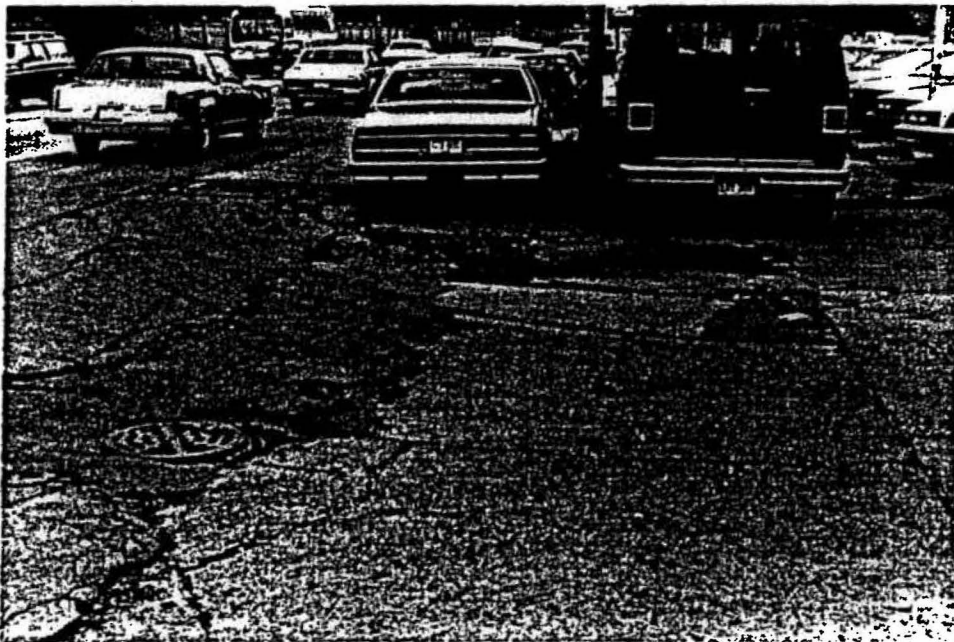
PHOTO C-2 Aged and deteriorated paving.
