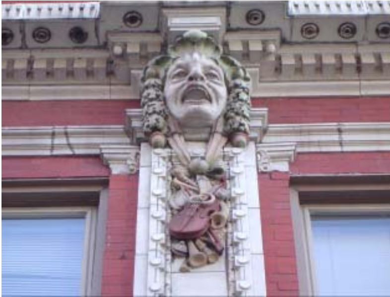
The Village Theatre (originally the Germania Theater) is heavily-ornamented with terra cotta, replete with German symbolism.
