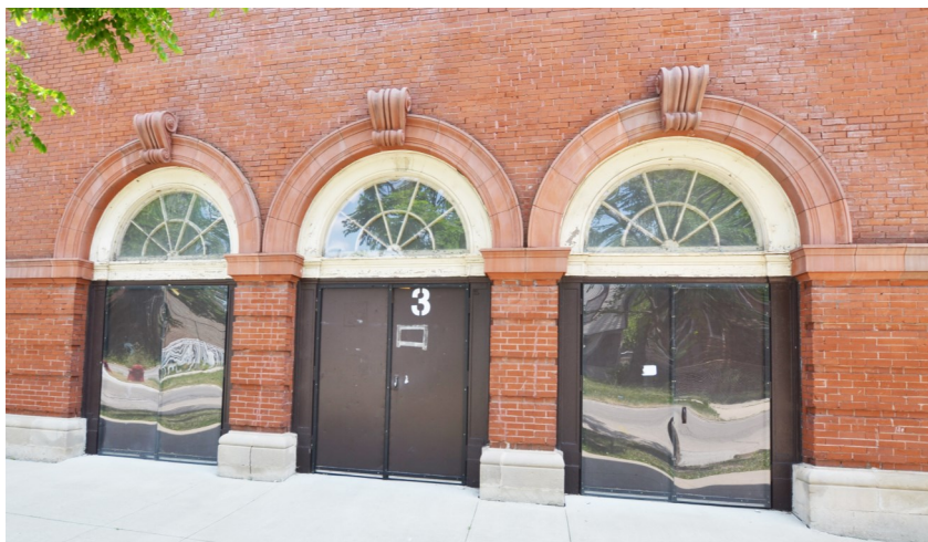
The 1923 addition has fine examples of Classically-inspired ornament. At left is shown a trio of entrances on the west elevation that lead to auditorium. Each is bordered in unglazed terra cotta and features a prominent keystone in the shape of a scroll.
