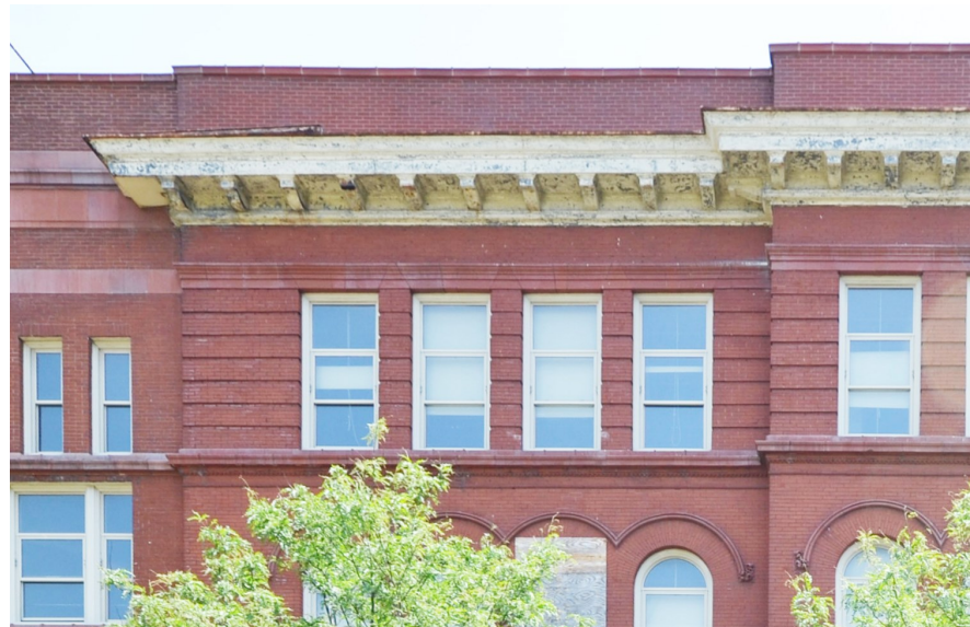
Right: The 1900 addition is similar to the 1894 section, but it includes a third floor with Classically-inspired details. Rusticated brickwork and a large metal cornice top the addition.
