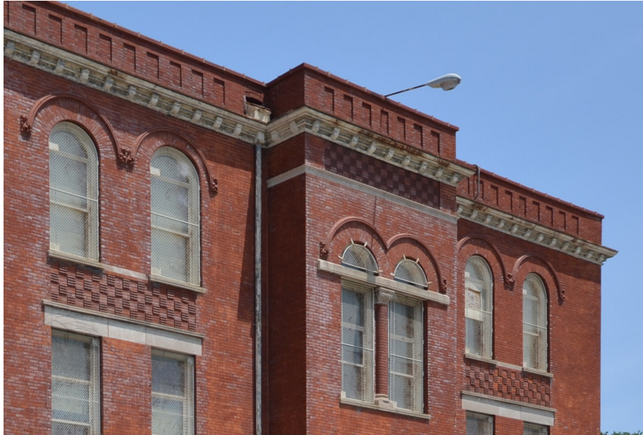
Left: The south elevation of Fiedler's 1894 building features decorative molded brick and fine arched terra cotta hood molds with foliate returns. The central bay features a twin stairwell window with a brick column as a mullion.
