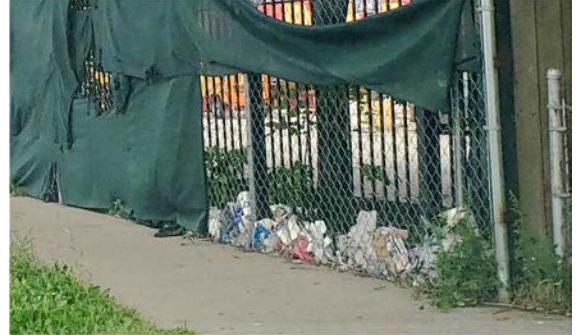
2019 Please address torn fence coverings and trash
